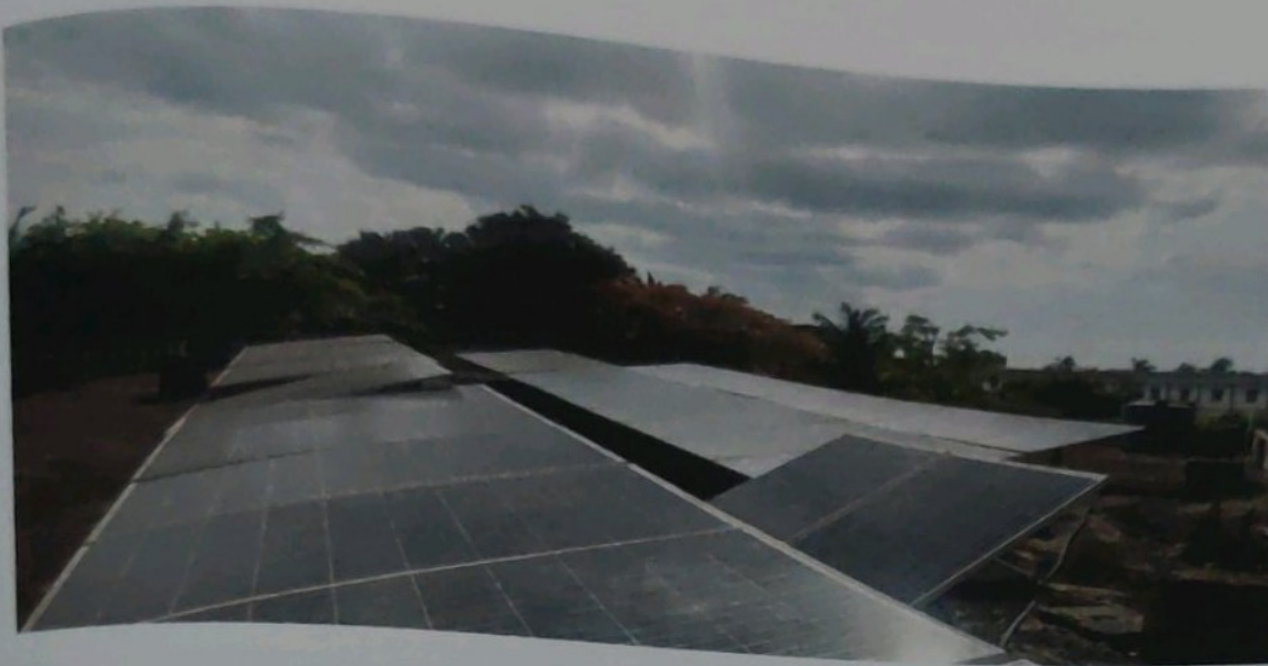
Solar Panels on the Rooftop of main Building
